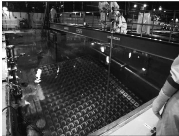
Fig. 4. PWR Spent Fuel Storage Pool.
