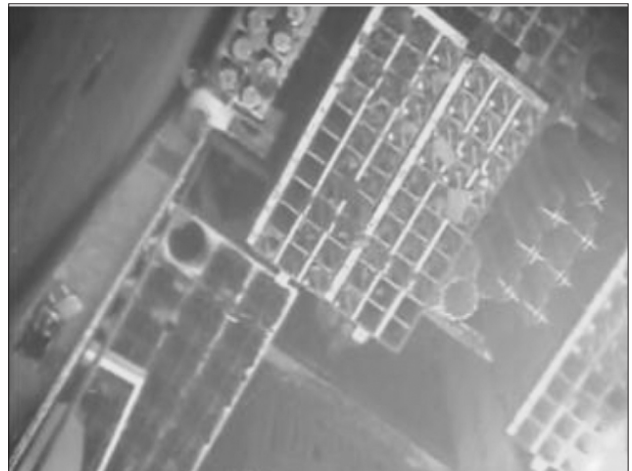
Fig. 1. View of Spent Fuel Storage Pool after Hydrogen Explosion at Fukushima Plant Unit 4(1).
