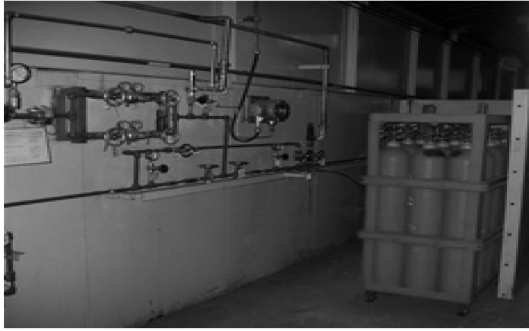
Figure 1. Interior system of storage & supply facilities of hydrogen gas.
