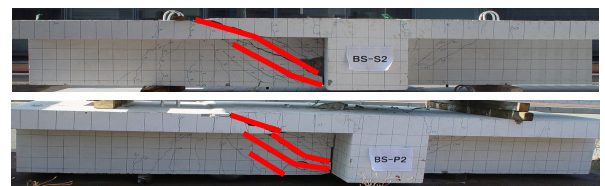
Fig. 7(b) Comparison with failures according to anchored place of hanger bars in designed ledger to simple supported beam
