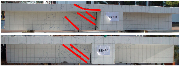
Fig. 11(b) Comparison with failures according to applied loads at any critical section for shear design
