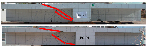
Fig. 6(b) Comparison with failures according to anchored place of hanger bars in designed ledger to composite beam
