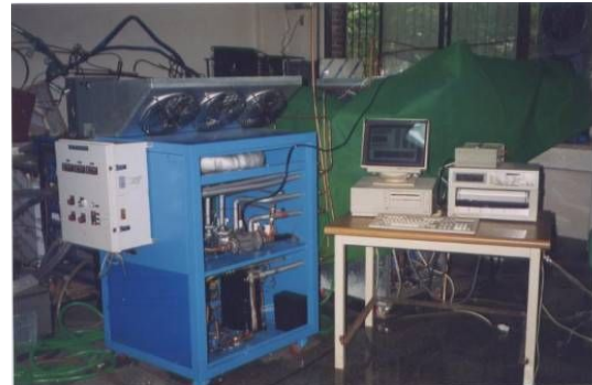
Figure 4. Experimental equipment of heat pump system (3PS).
