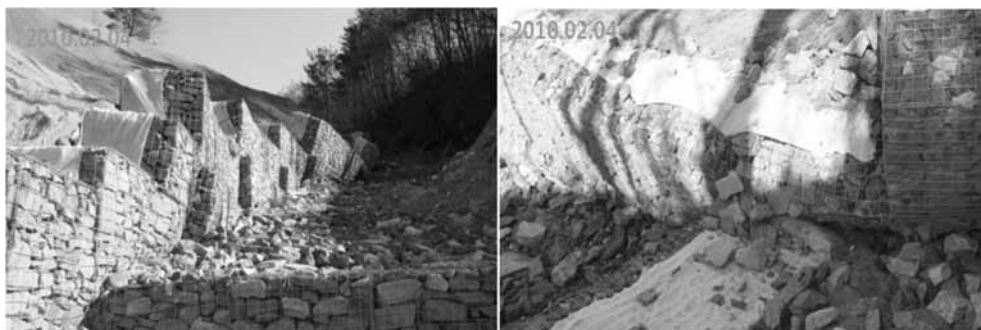
(a) Toppling failure of gabion walls
