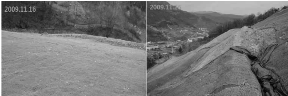
Fig. 20. Deformation of the cutting slope after 4 months.
