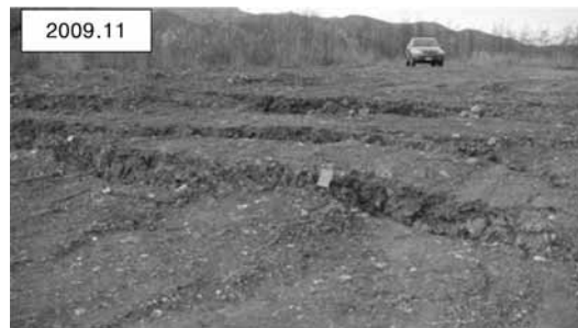
Fig. 16. Tension cracks after covering work.
