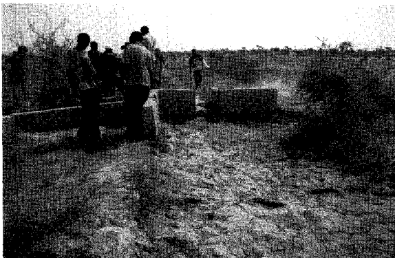
Structure & Silted Canal
