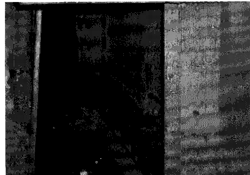
(a) Corrosion in cross beam
