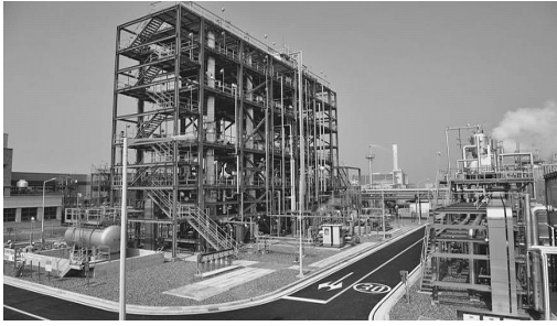
Fig. 1. Overview of 10TPD DME Demo Plant in KOGAS.
