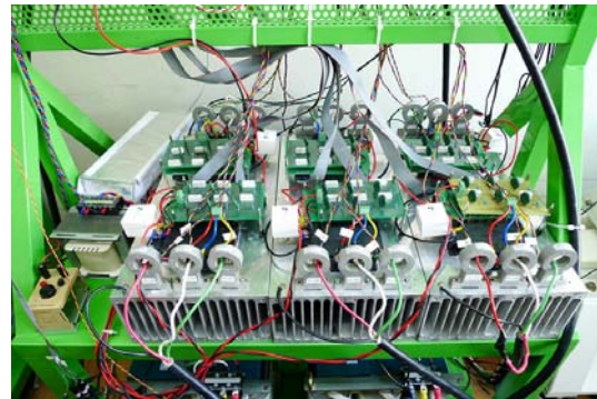
(c) The power converter.
