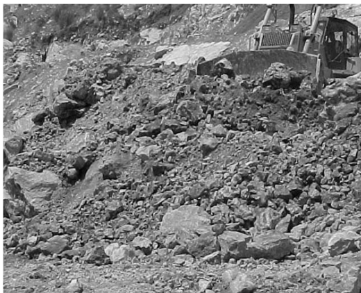
Fig. 2. Tight muck piles being pushed by the dozers from top of the bench.
