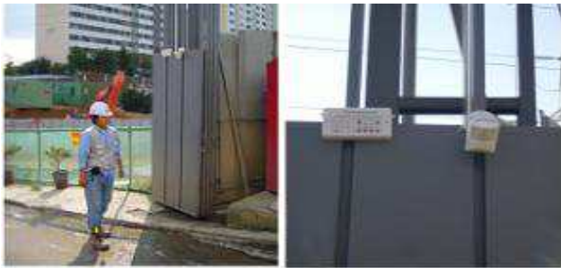
Figure 1. Installation place : Zone A
