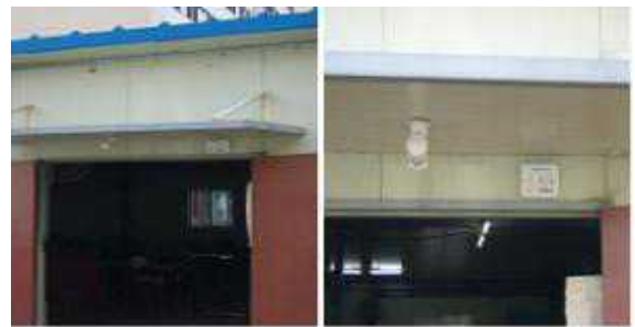
Figure 3. Installation place : Zone C
