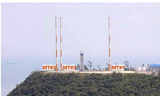
Fig. 10. Lightning Protection Towers around Launch Pad
