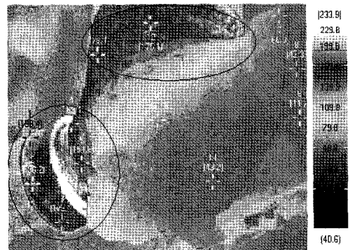
Fig. 6 Result of thermal image measurement for AC-HV-015A valve
