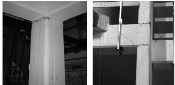
Fig. 15 Bond slip at column ends of the test frame
