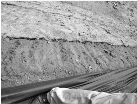
Fig. 9. Tension crack by toppling failure.
