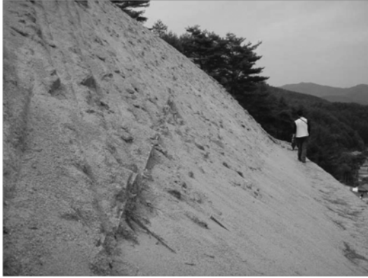
Fig. 5. Shallow failure at upper part of 4th berm.
