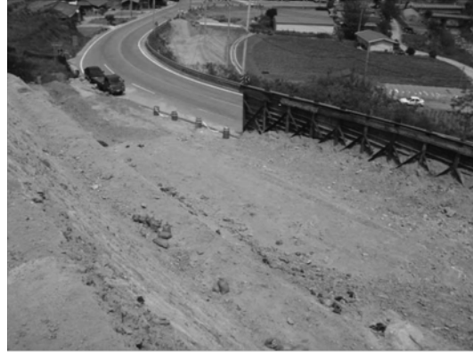
Fig. 6. Non-existing rigid rock body at STA.0 + 380~0 + 420.
