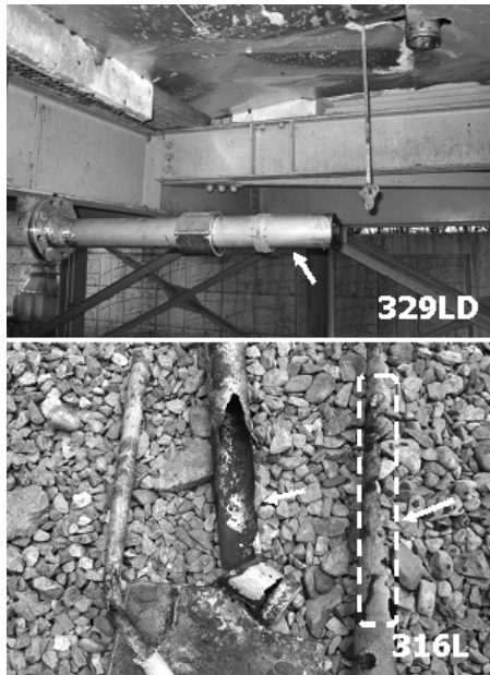
Fig. 4 Comparison of corrosion properties between 329LD and 316L for slurry pipes in regional power plants
