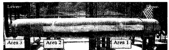
(a) Area 1, 2, 3 in the elbowed pipe
