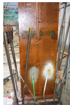
(b) connection between ground wire and steelwork
