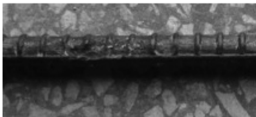
Fig. 1 View of steel corrosion
