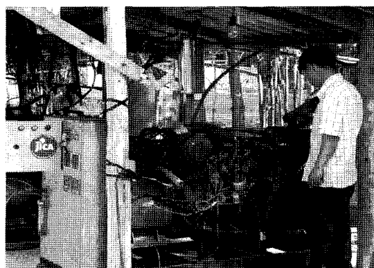
Fig. 2 Power generation system using biogas fuel for this research in the program of JICA - SUPREM project.
