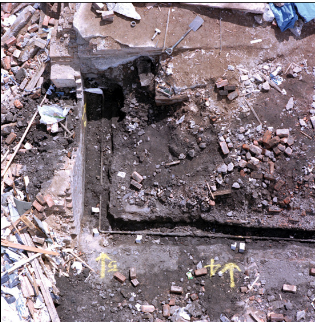
Fig. 10. The corroded pipe which leaked LPG causing the explosion.
