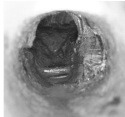
(a) Exposed wires prestressed 66% of tensile strength
