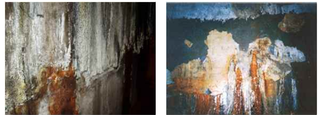
(a) Corrosion of sulfuric acid (b) Corrosion of chlorine
