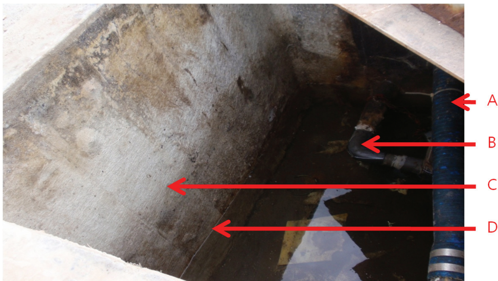
Figure 2. Water pipes and waste pipes in the same place with the trace of high water level mark.
