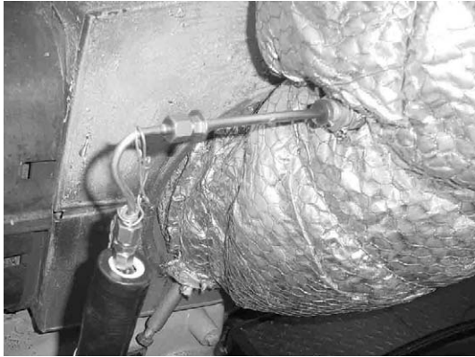
Fig. 8 Installing of probe for Smoke analyzer
