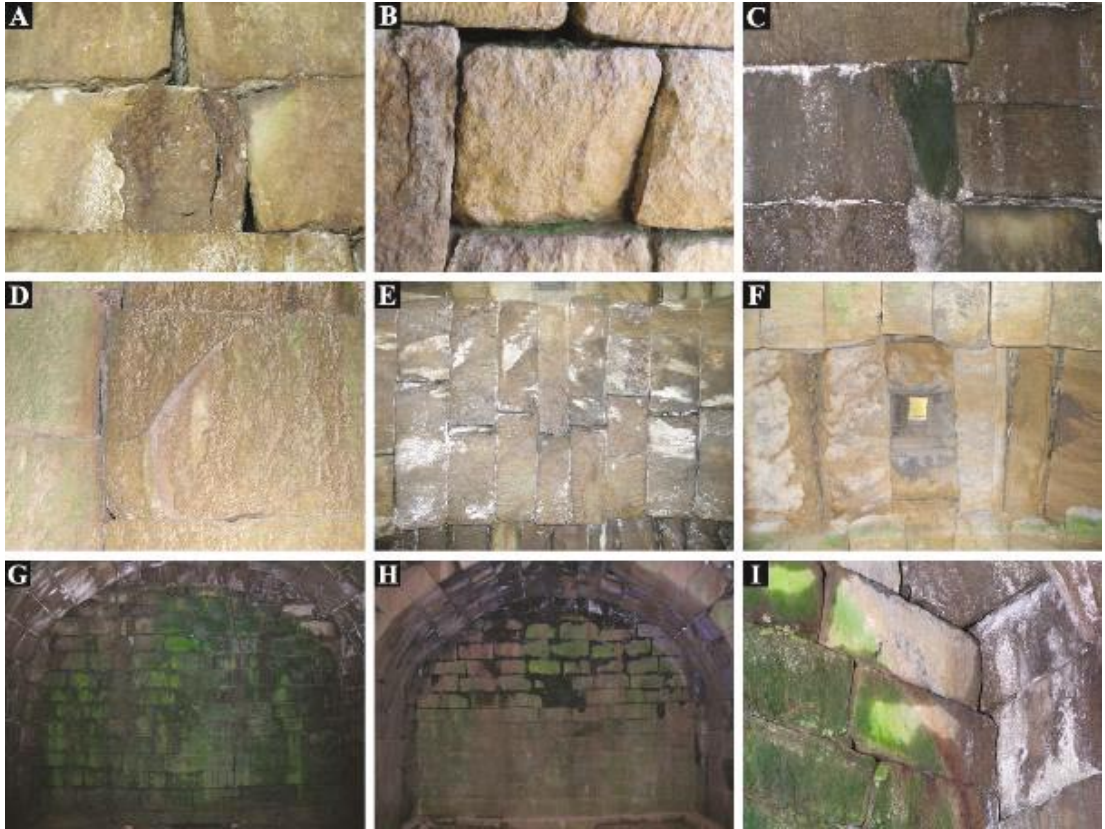
Figure 4. Occurrence of individual weathering forms in the Gyeongju Seokbongp. (A) Cracks of an interior arch store. (B) Disjoining due to irregular array between rock blocks. (C) Breaking-out of an arch store. (D) Exfoliation parallel to the store surface. (E) Efflorescence on the arched ceiling. (F) Considerable brown and dark-gray discoloration around the ventilation ducts. (G) Distribution of biospecies on the north wall during summer. (H) Distribution of biospecies on the north wall during winter. (I) Different distribution of biological colorization between lightened and shaded area.
