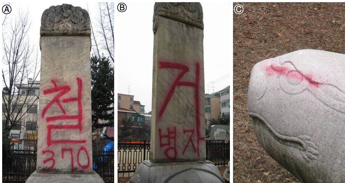
Figure 1. Damaged aspects of the Samjeondobi Monument. (A) Front side. (B) Back side. (C) Tortoise pedestal.
