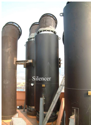
Fig. 10 Resonator type silencer installed in exhaust stack
