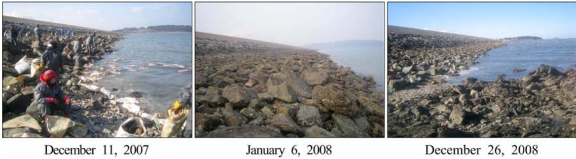
Fig. 14. Change of oil-polluted Iwon tide embankment by the Hebei Spirit oil spill incident.
