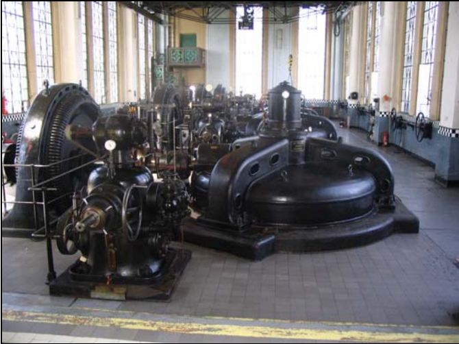
Fig. 1 Powerhouse - 4 original units in line
