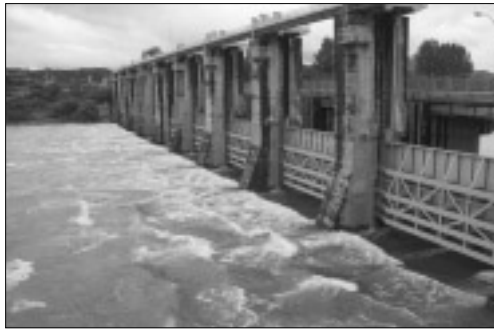
(a) Floodgate of control place
