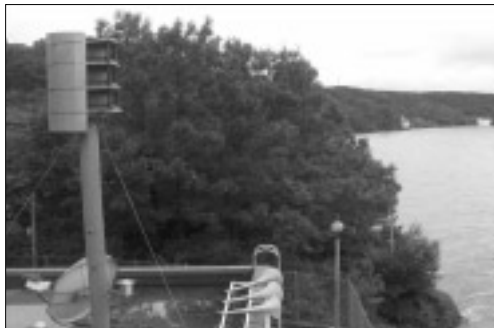
(b) Speaker of alarm office in control place
