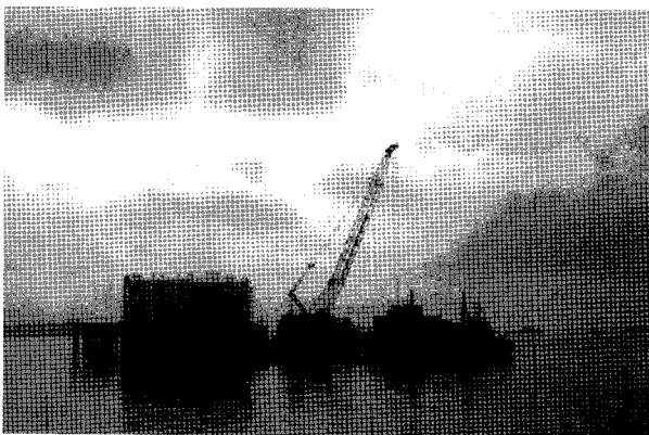
Fig. 7 Uneven settlement after placing the PIER 4 caisson
