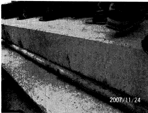
Fig. 1 Crack in track slab
