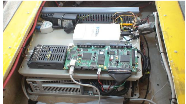
Fig. 2 Data acquisition system
