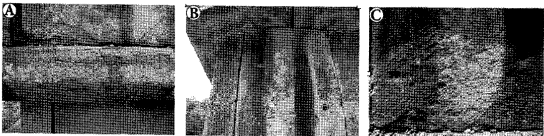
Fig. 3. Representative weathering of host rocks for the stone Buddha and Shrine. (A) Physical weathering by irregular shaped cracks of the roof rock in southern basement. (B) Biological weathering by lichen and algae of the face rock in western basement. (C) Chemical weathering by surface oxidation of the face rock in western basement.
