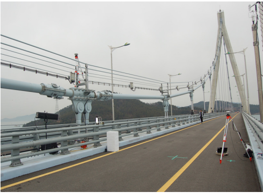
Fig. 3 The DGPS system installed on So-rok Bridge
