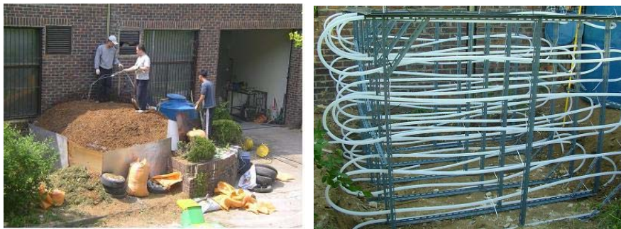
Fig. 2. Fermenting beds and pipe installation (plate type) for heat exchanger.
