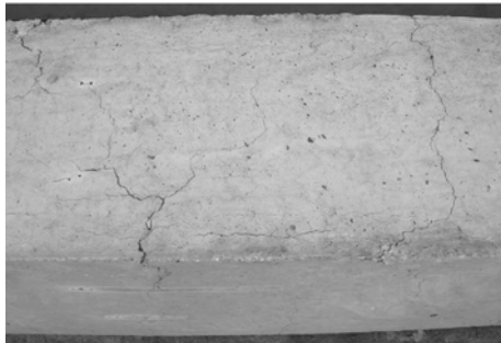
(b) Surface cracks of specimen S61
