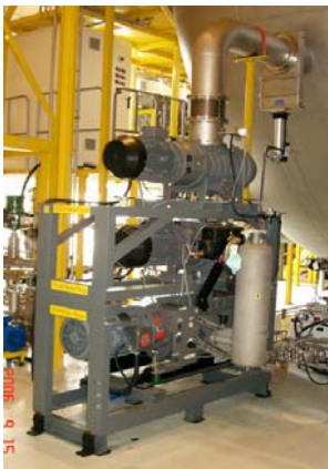
Figure 7. Primary pump system
