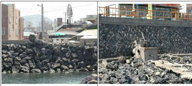
Photo 3. Yongduam area with ocean water pumping system in Jeju city.
