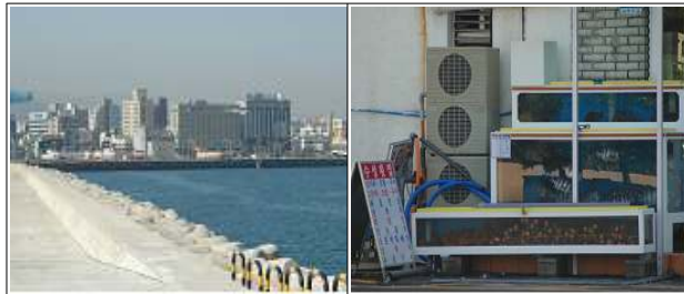
Photo 2. Topdong area with ocean water pumping system in Jeju city.
