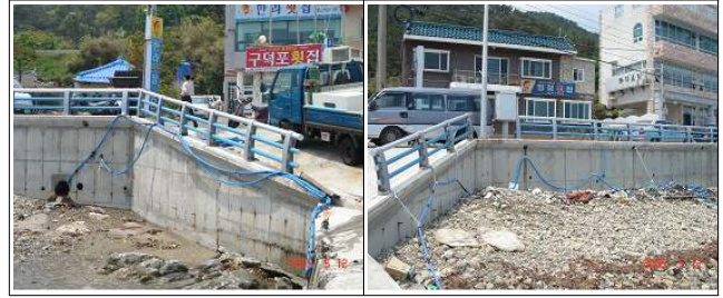
Photo 9. Gudeokpo area with ocean water pumping system in Busan city.
