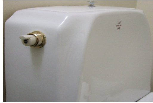
Fig. 5. Water saving toilet stool.
