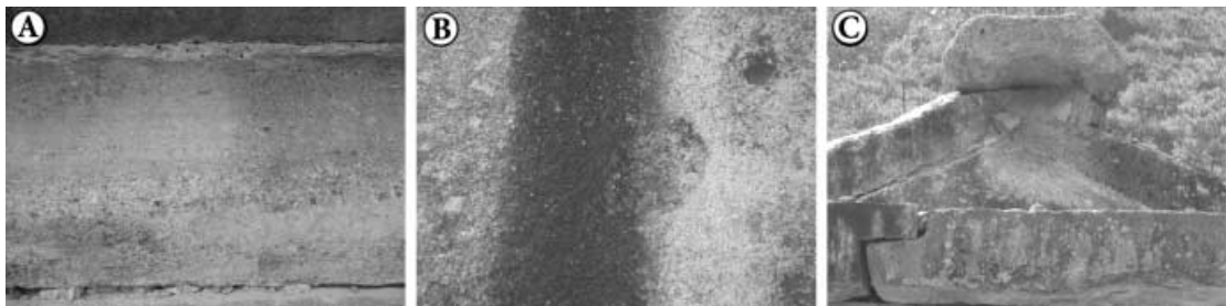
Figure 8. Representative chemical weathering of host rocks for the stone Buddhas and Shrine. (A) Northern under base rocks show yellowish brown discolorations developed on surface, (B) Western wall rocks show dark discolorations developed on surface, (C) Western roof rocks show white discoloration.
