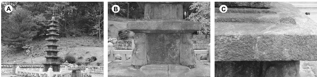
Figure 1. (A) Current state of the Daewonsa temple stone pagoda. (B) Stone surface coated with reddish brown discoloration due to oxidation of rock properties. (C) Basement roof stone rejoined using cement adhesion.
