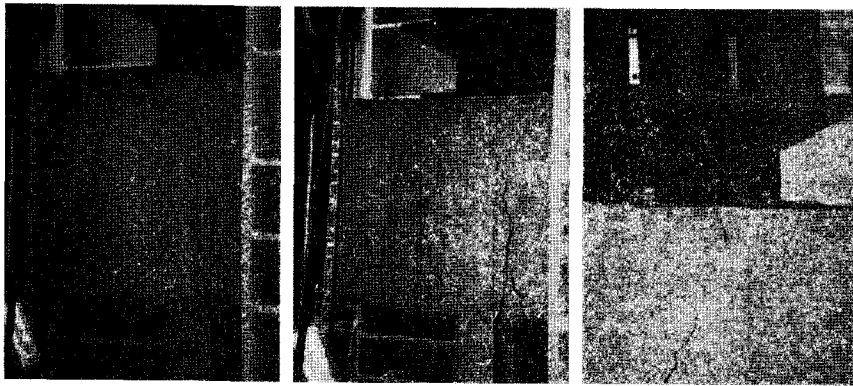
Fig. 9. Bending crack status at the time of imminent failure,
