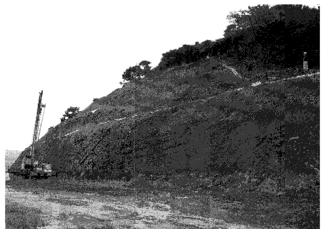
Figure 3. It shows a road construction work cutting hillside off at the edge of breeding site of the egrets and herons, Palhyunri, Daegu
