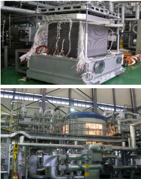
Fig. 2 75kW test set-up
