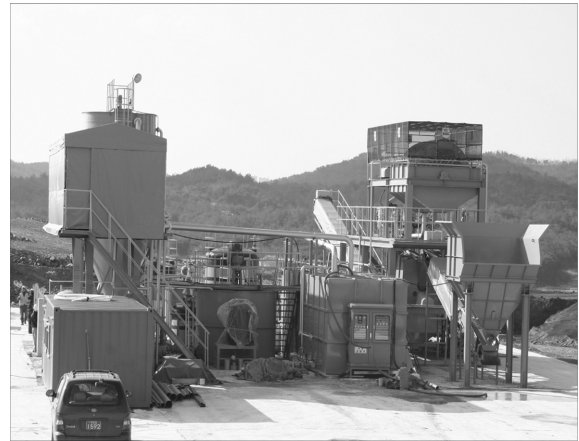
Fig. 1. full scale soil washing plant.
