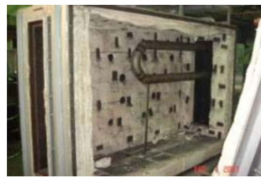
Fig. 4 The inside of test furnace
