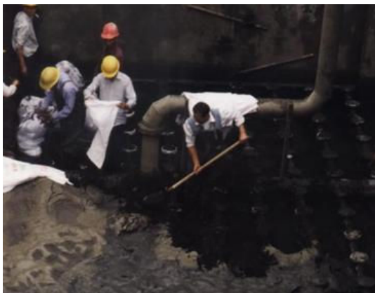
Fig. 7. Accumulation of sediment in aeration basin due to poor performance of grit chambers
