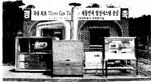
Fig. 5 60 kW MGT grid-connection model(KEPCO KEPRI, Daejeon)
